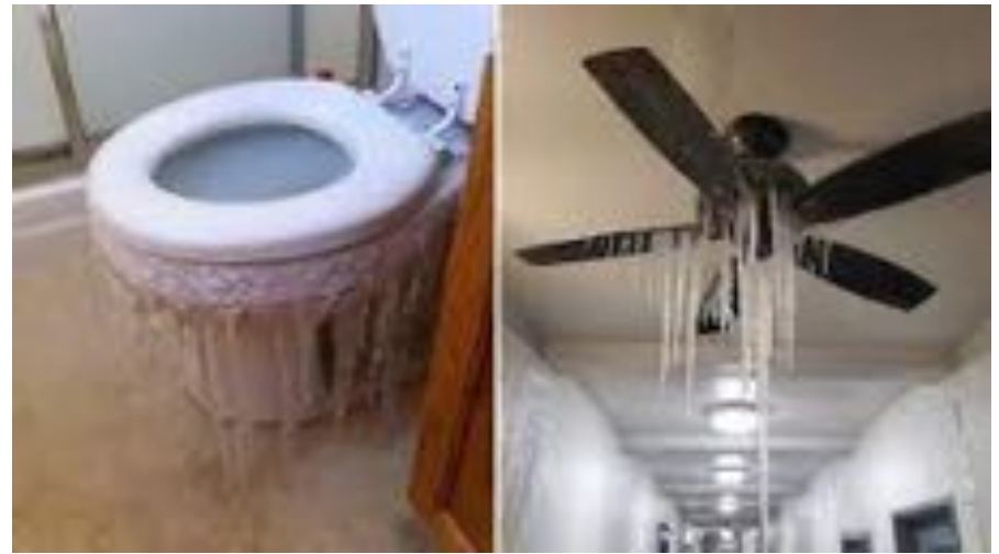
Pipe bursts resulted in water outages and destruction; particularly in older homes
